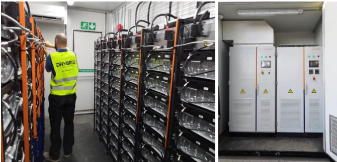
Figure 2: Cheetah Plains Battery Container
