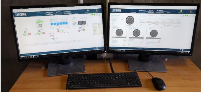
Figure 4: DHYBRID UPP SCADA System for Real-Time Monitoring
