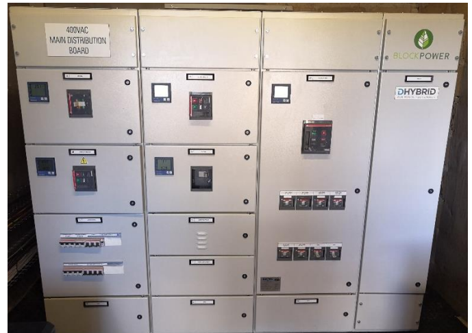
Figure 3: New 3-Phase Distribution Board with motorized Breakers
